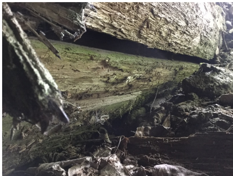
Horizontal crack in left bank sill
