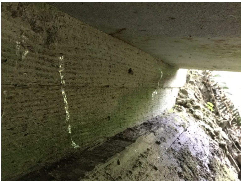
Downstream left bank timber condition
