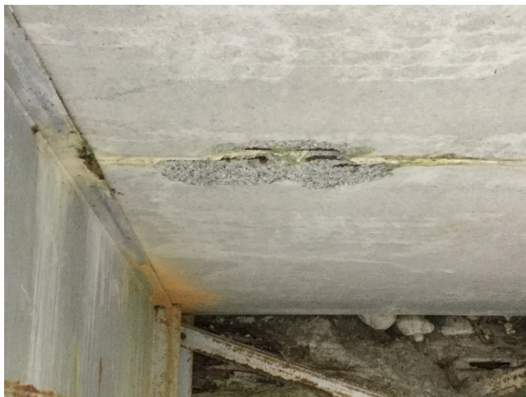
Damage noted to panel 1 and 2 at right approach
